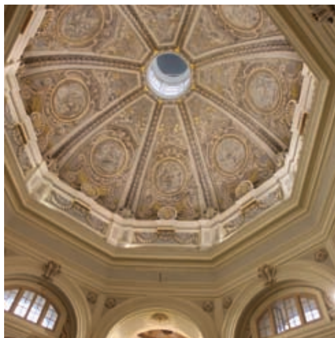
Completion of the restoration works of the cupola of St. Catherine of Italy
